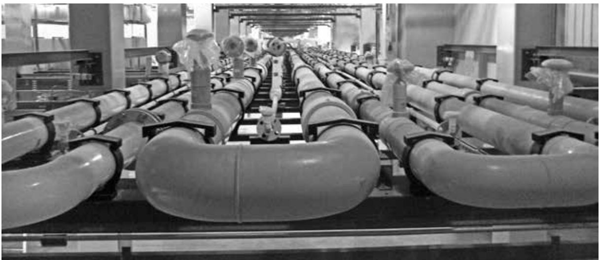
Figure E.7: High purity piping system installed with AGRU pipe clips.
